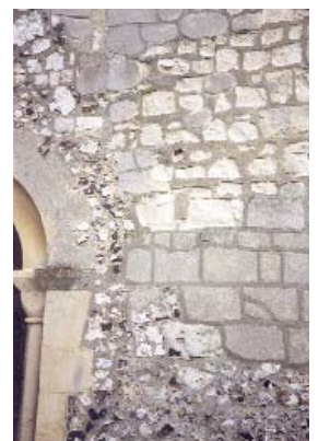
Inappropriate cement mortar repointing has damaged the soft limestone irreversibly
